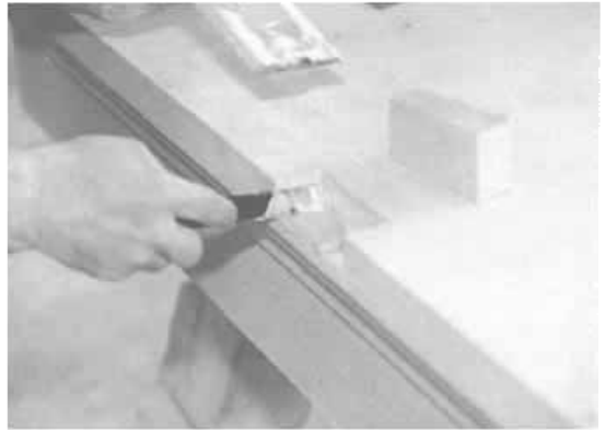
4 Make certain that the contact surfaces of repair stone will fit the slot. Then, butter the squared hole with epoxy mixed for the purpose.
