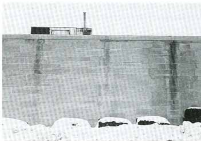
Leaking connections in this metal coping collect water and dirt which flood over the stone below in a concentrated flow.
