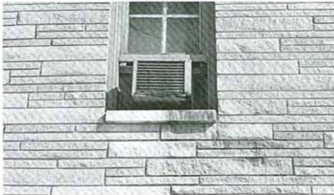
Lack of maintenance on this air conditioner has produced a badly stained sill and other stones in the splitface wall below.
