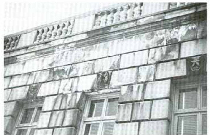
A badly leaking roof caused this eyesore. When the leaks were repaired, the efflorescence cleared up within a few months.
