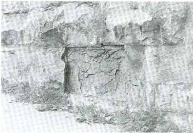
Typical sheeting in exfoliating limestone at the base course of a retaining wall (ca. 1880). The stone is sluffed off in thin layers. Compare to exfoliation in concrete shown in the following photograph.
