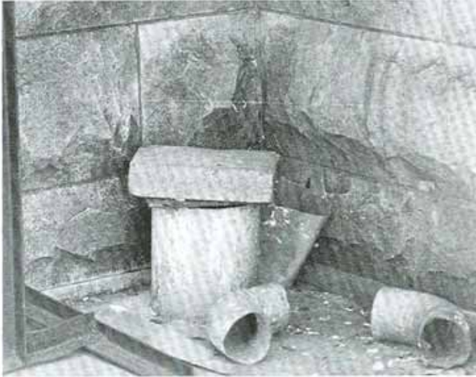
This corner area provides the necessary conditions for a growth of moss. Other vegetable growth may develop with the added nutrients of droppings.
